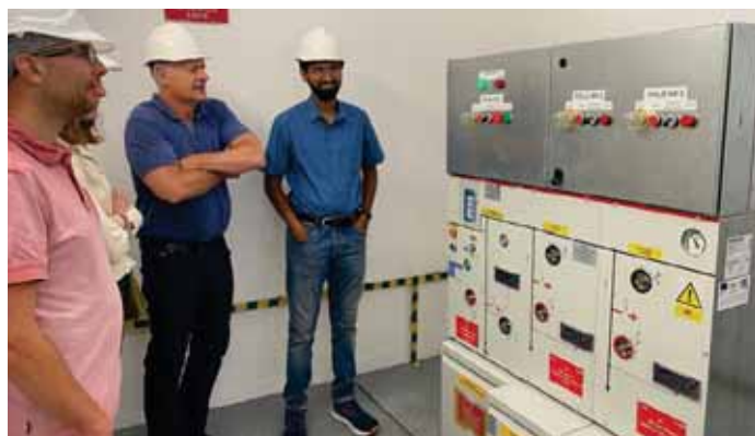
Fig. 7: Updated substation for automated control in Sopot, Poland
