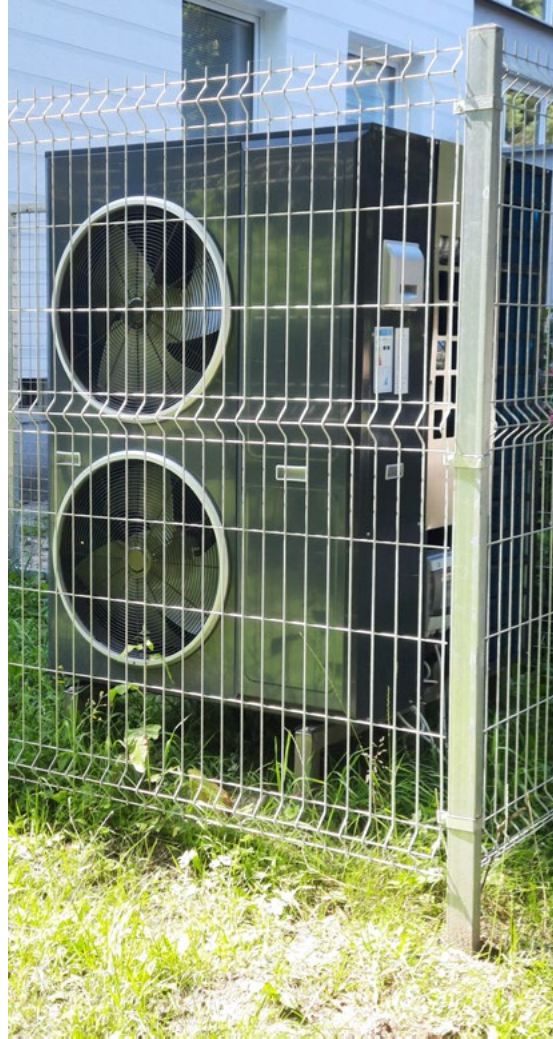
Fig. 1 Heat pumps in front of the Mickiewicz 59 block of flats (K. Bogucka-Bykuć, IMP, 2024).
