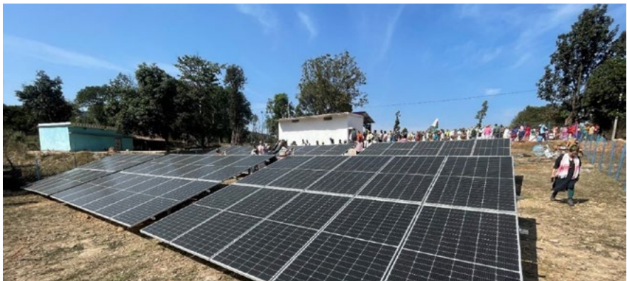
Fig. 6 PV installation in the Barubeda Village (R. Sinha, Aalborg University, 2024).
