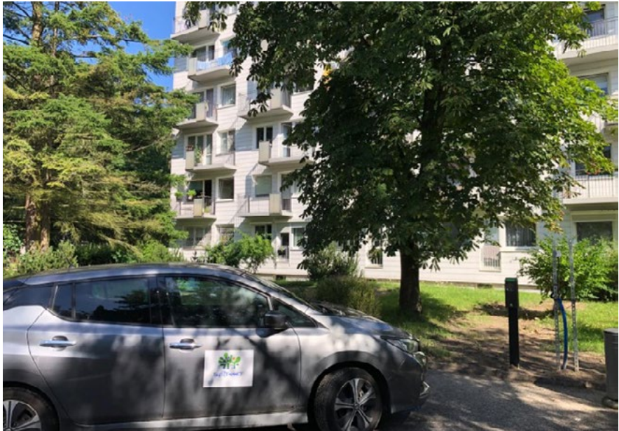
Fig. 2 One of the EV chargers installed at the Mickiewicza Housing Association and Nissan Leaf used for tests (S. Bykuć, IMP, 2024).
