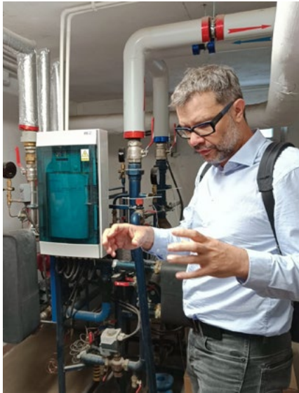
Fig. 6 Sebastian Bykuć, IMP PAN, KEZO Research Centre, depicting works related with the modernized heat node for DHW production at the Polish site (Joanna Ptak, Energa Operator, 2023).
