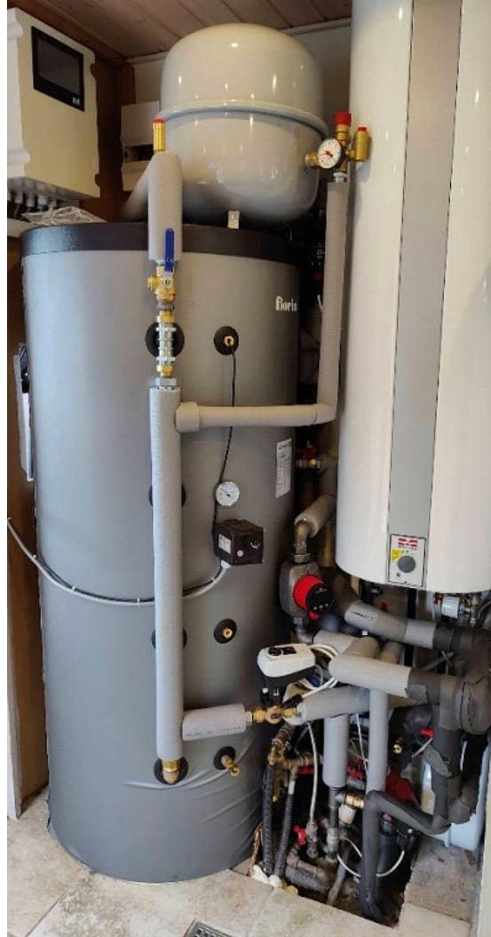
Fig. 1: Example of the upgraded installation at a testhost (Neogrid Technologies, 2023).
