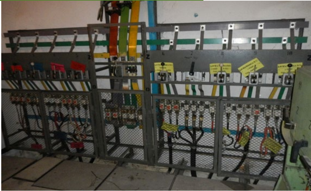
Fig. 1. Interior of the T-2846 Mickiewiczza Sopot secondary substation BEFORE modernization (Robert Klein, Energa-Operator SA, 2023).
