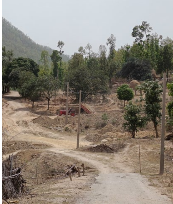
Fig. 3 Metering and household wiring activity in Borakhai (IIT Bombay, 2023).
