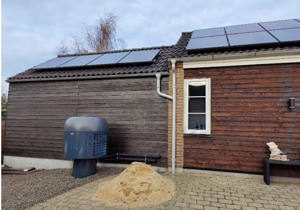
Fig. 2: The outside installation of a testhost - with both heat pump and PV system (Neogrid Technologies, 2023).
