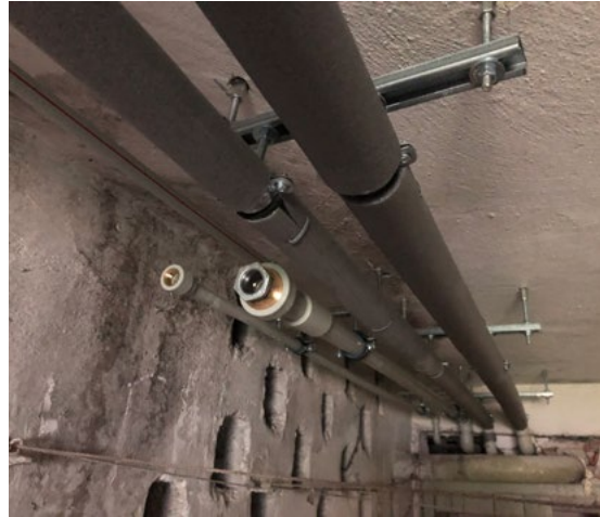
Fig. 3 DHW distribution pipes (Sebastian Bykuć, 2022)
