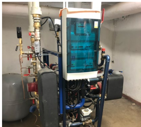
Fig. 4 The modernised heat node with DHW production (Sebastian Bykuć, 2022)
