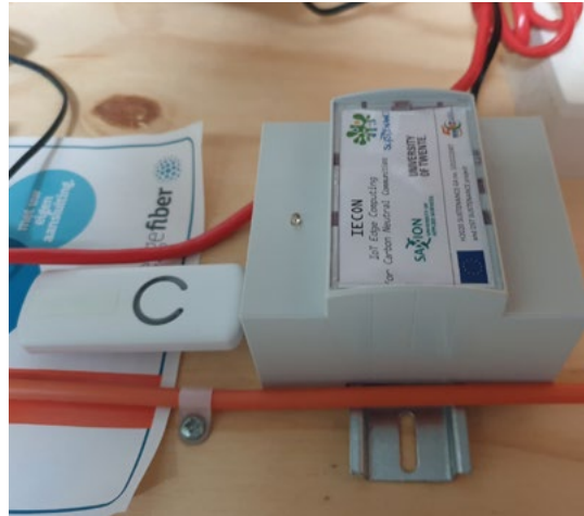
Fig. 1 IECON system installed at Vriendenerf
