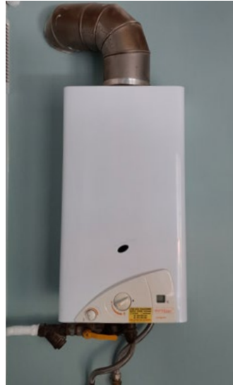
Fig. 5 Individual gas boiler (used for preparation of DHW)- to be dismantled in late summer 2022 (Sebastian Bykuć, 2022)
